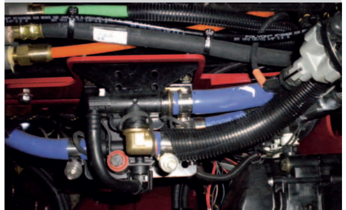
Mounted coolant line component
